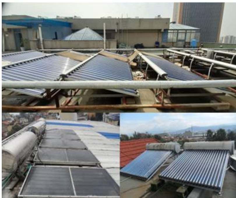
Figure 4-10: Some of SWHs systems in hospital and health specialty centers
