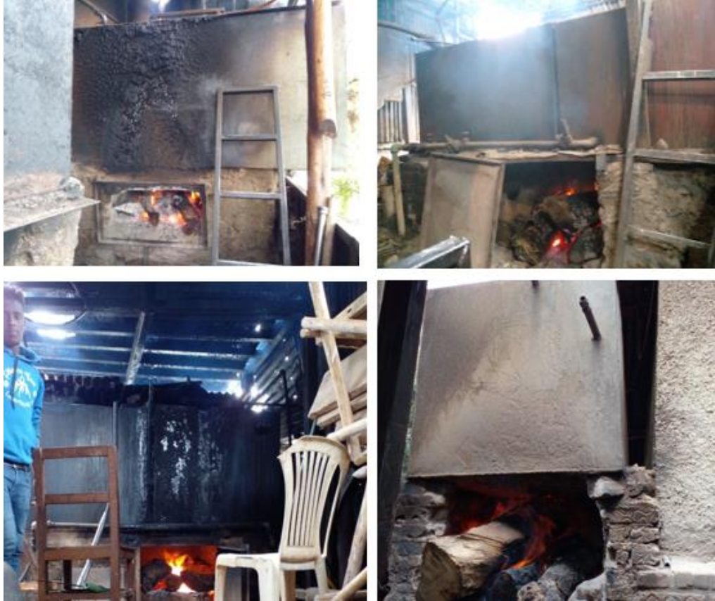
Figure 4-51: Fire wood water boiler at shower houses
